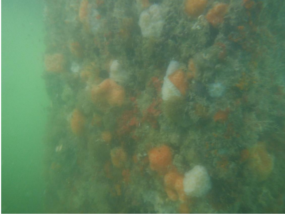
Photo 15: Typical live bottom on existing bridge piles
