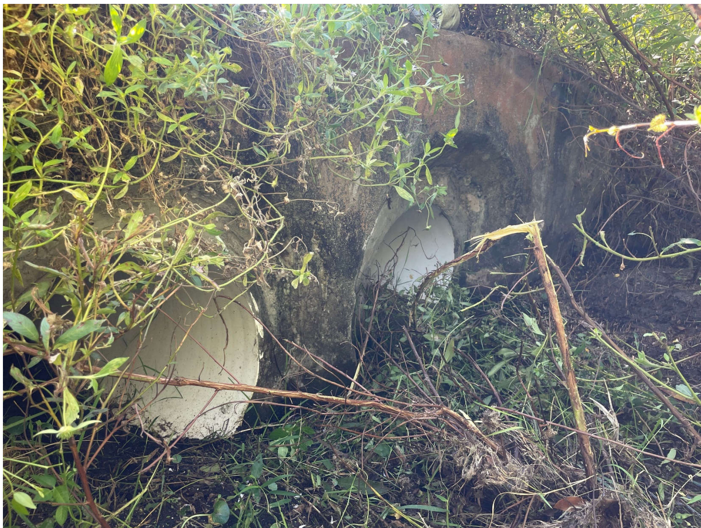
Double barrel culvert on the west side of US 27. Photo taken facing southeast.
