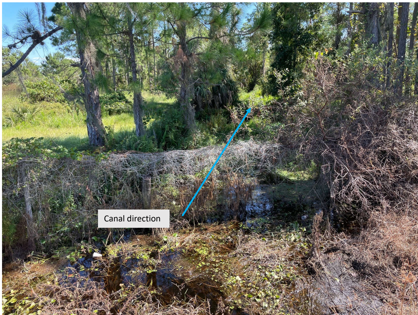
Canal approaching box culvert from southeast on the east side of US 27. Photo taken facing southeast.
