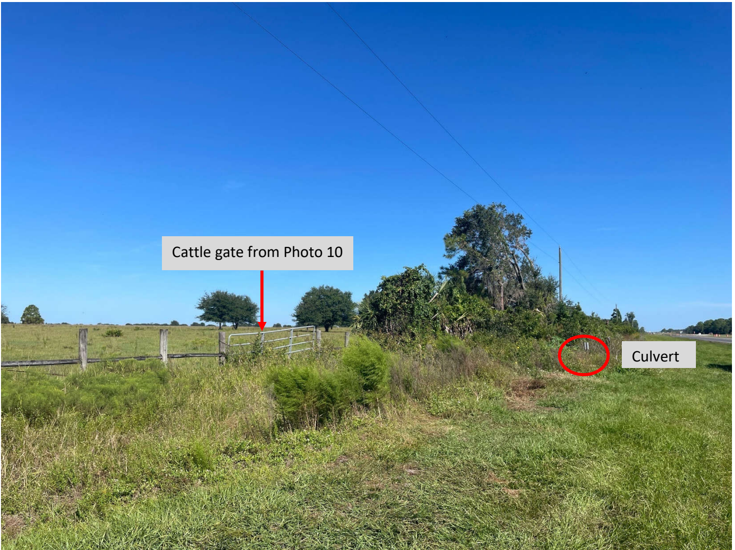
View of box culvert in relation to adjacent cattle gate on the west side of US 27 facing north.
