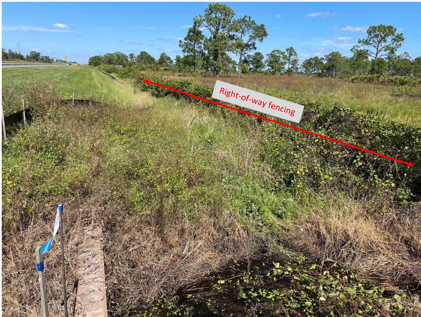
North facing view from east side of US 27 at box culvert. Vine-covered right-of-way fencing extends to north.
