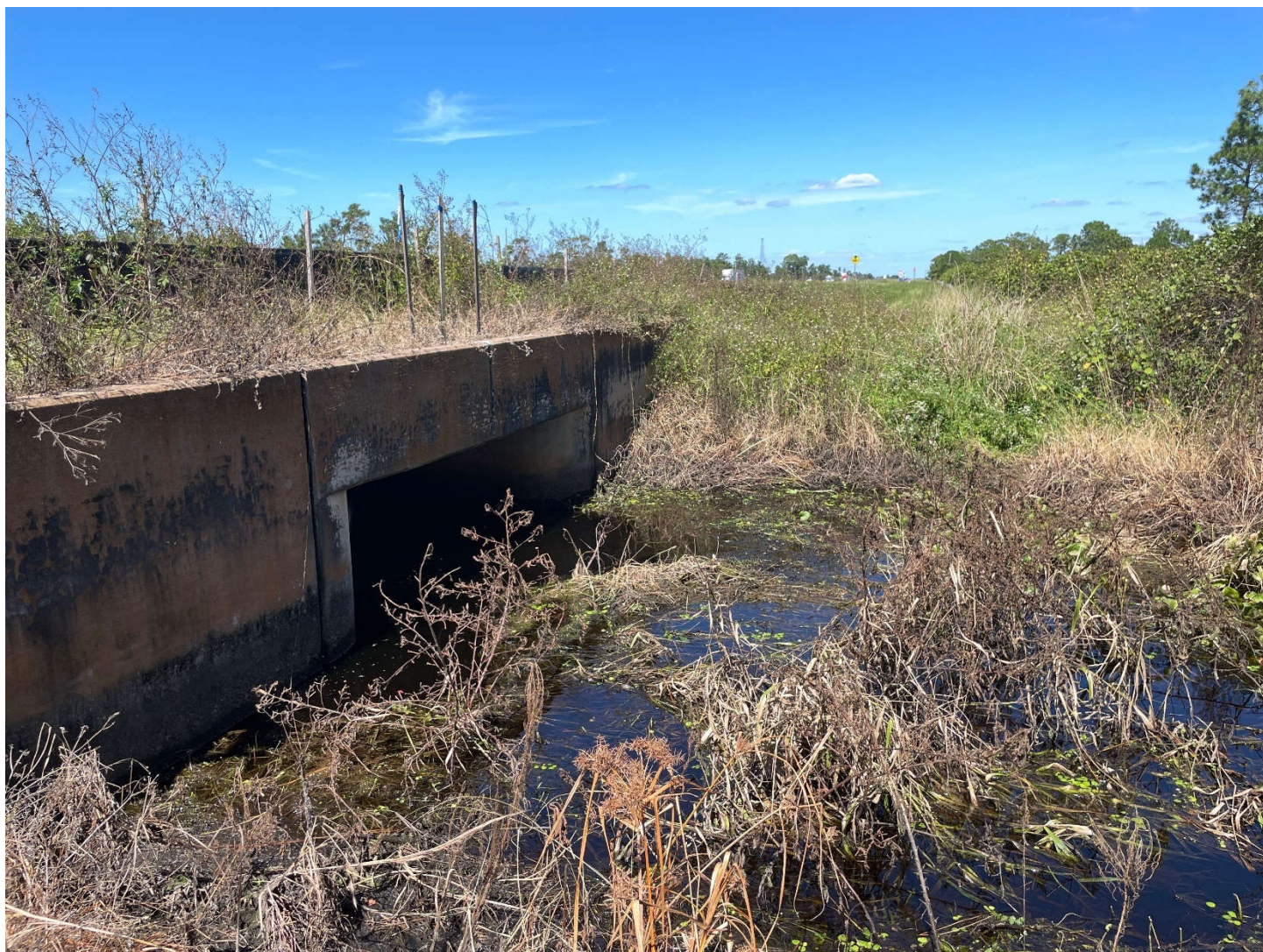
Existing box culvert on east side of US 27. Photo taken facing north.
