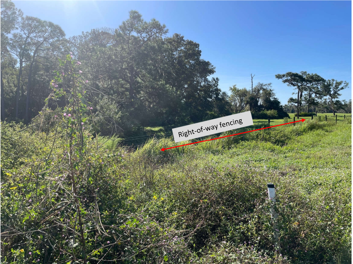
View from top of headwall facing southeast on east side of US 27.
