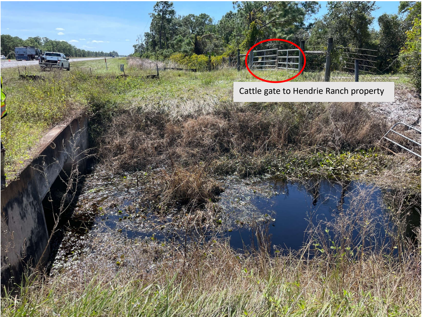
South facing view on west side of US 27. The adjacent cattle gate and unpaved driveway/road can be observed to the south of the canal.
