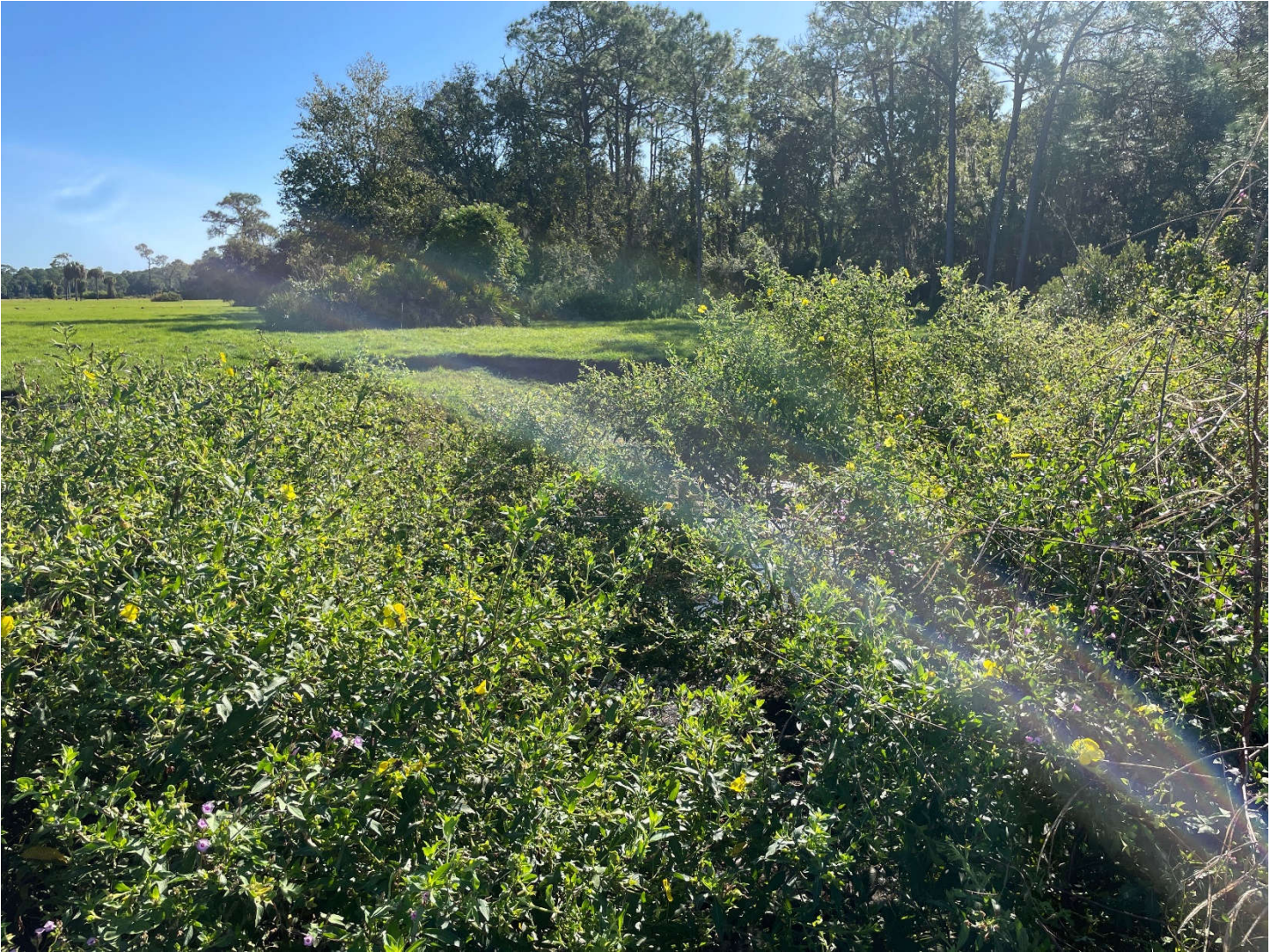
View from top of headwall at culvert facing east on the east side of US 27.
