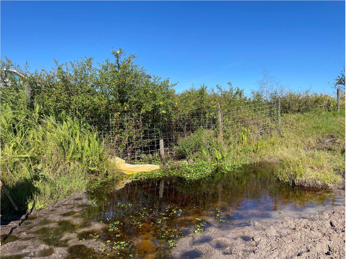
View of culvert from east side of US 27 on the east side of the right-of-way fencing northwest.
