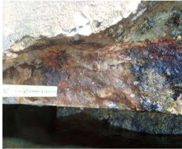
Figure 2.2.3 Typical Corrosion at Footing
