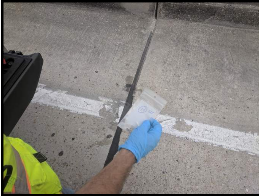
Photograph 13 View of Asbestos Homogeneous Area 4 – White Lane Paint – Roadway Deck (Sample Location 12).
