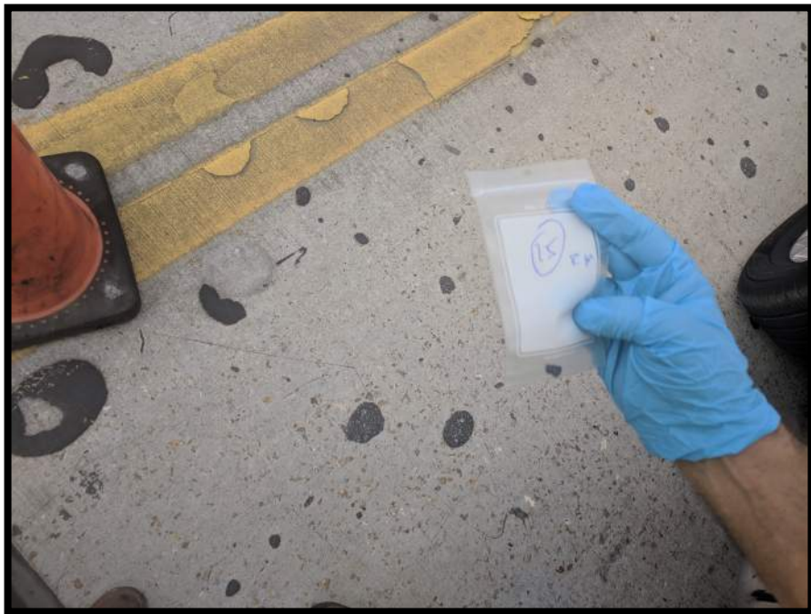
Photograph 16 View of Asbestos Homogeneous Area 5 – Reflector Mastic – Roadway Deck (Sample Location 15).
