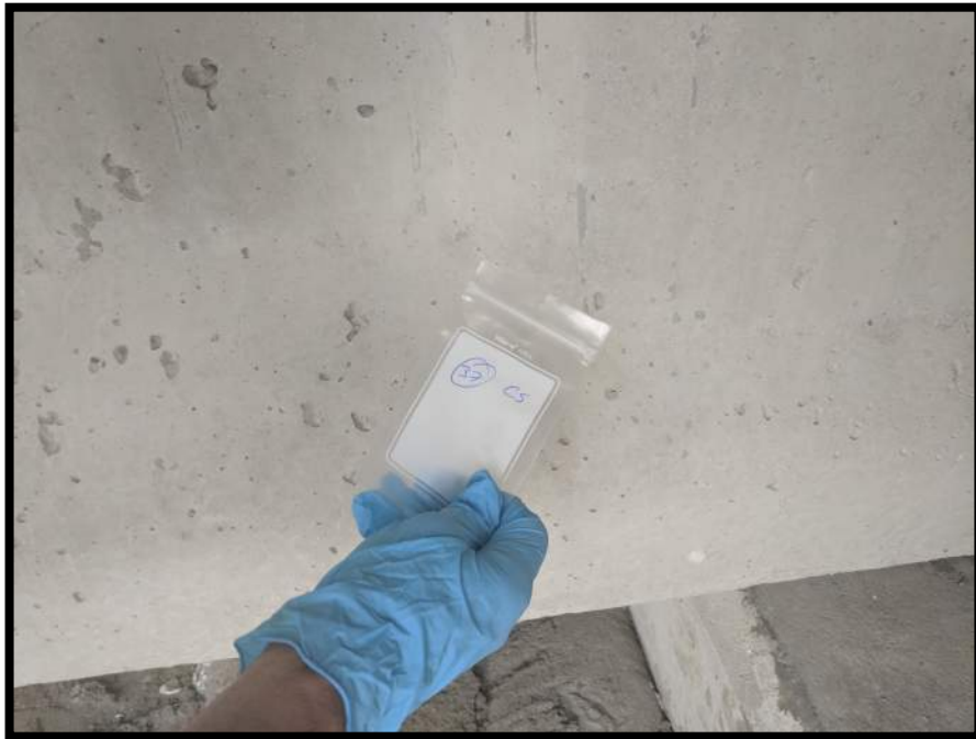
Photograph 38 View of Asbestos Homogeneous Area 13 – Concrete – Structural Beams, Abutments and Pilings (Sample Location 37).
