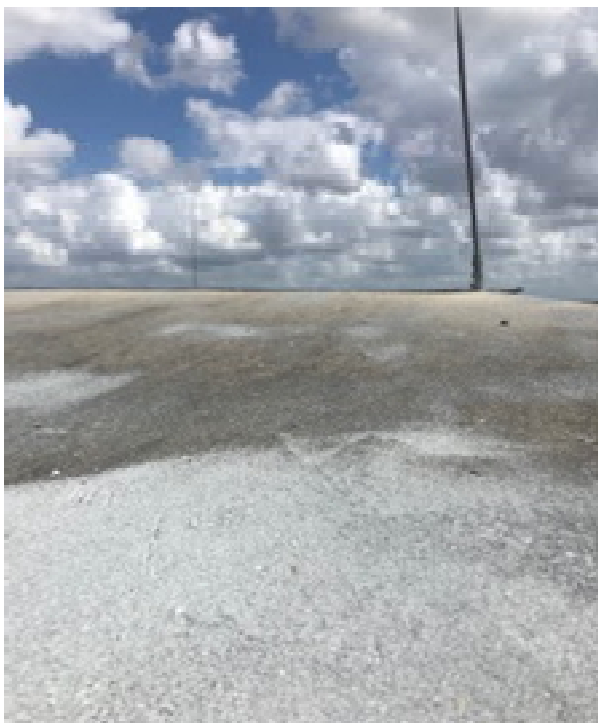
Photo No. 3- Non-Asbestos-Containing Class 5 Coating on Concrete Tender House Roof and Roadway Barriers
