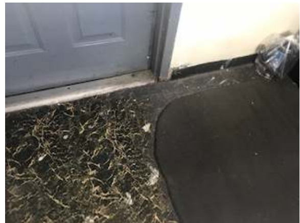
Photo No. 4- Asbestos-Containing Floor Tile and Adhesive in Tender House
