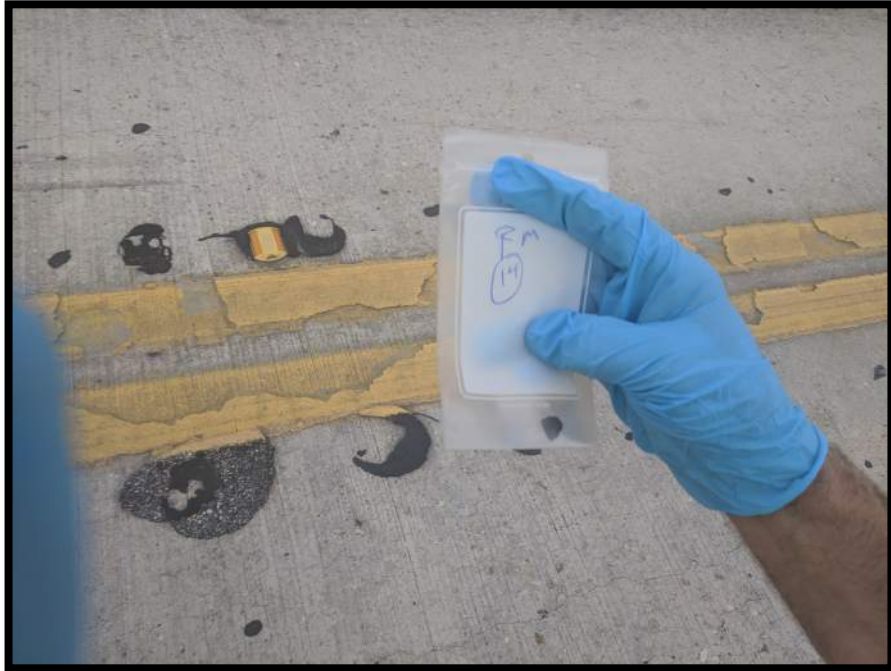
Photograph 15 View of Asbestos Homogeneous Area 5 – Reflector Mastic – Roadway Deck (Sample Location 14).
