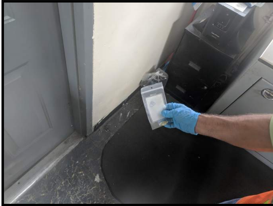
Photograph 33 View of Asbestos Homogeneous Area 11 – Textured Wall Paint – Tender House (Sample Location 32).
