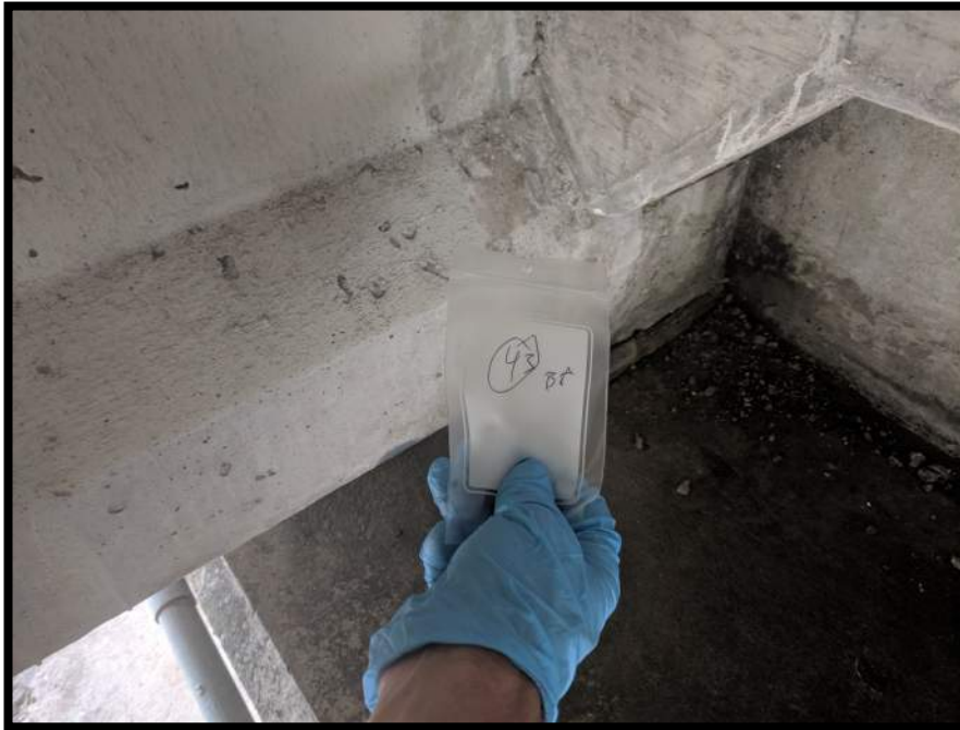
Photograph 44 View of Asbestos Homogeneous Area 15 – Bearing Pads – Beneath Bridge (Sample Location 43).
