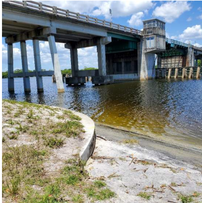
Site 21 – Wilson Pigott Bridge South side of river looking northwest View of tender house
