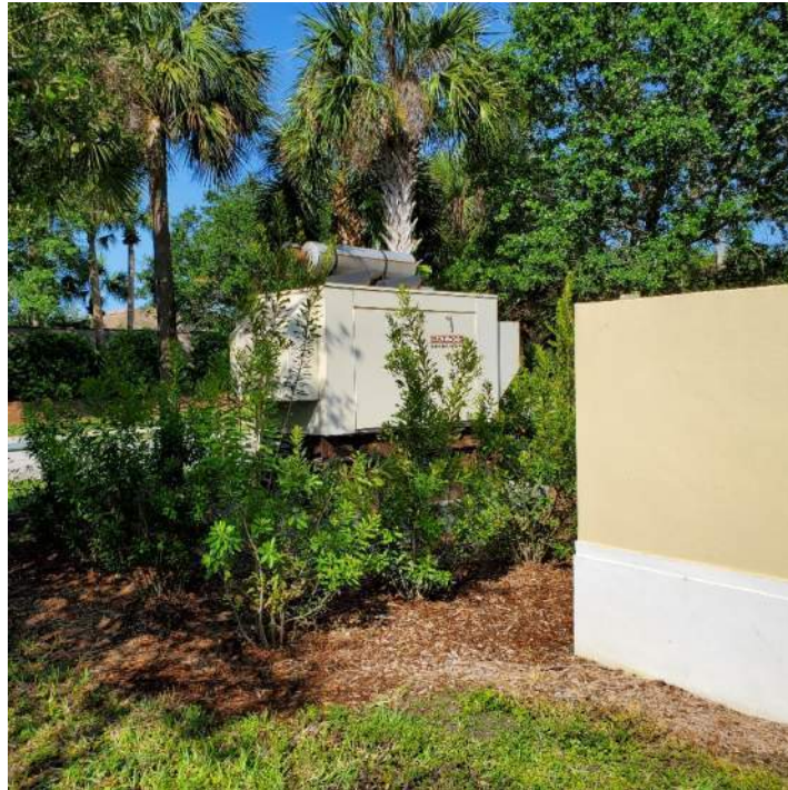
Site 3 – First Bank Emergency generator with base tank (diesel fuel)
