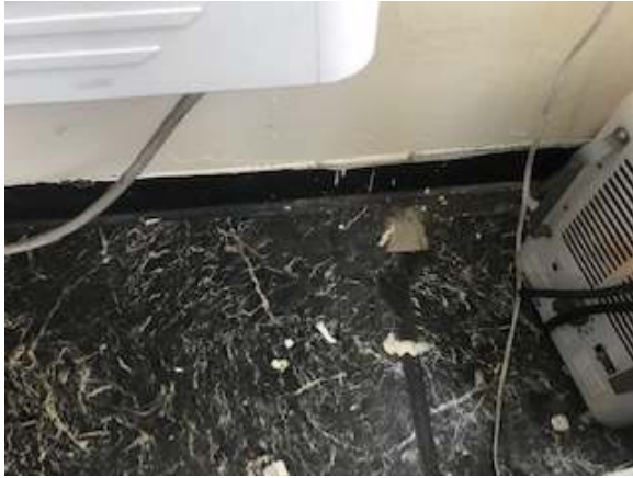
Photo No. 5 - Non-Asbestos-Containing Cove base in Tender House
