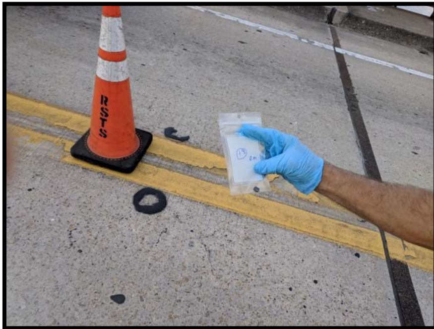
Photograph 14 View of Asbestos Homogeneous Area 5 – Reflector Mastic – Roadway Deck (Sample Location 13).
