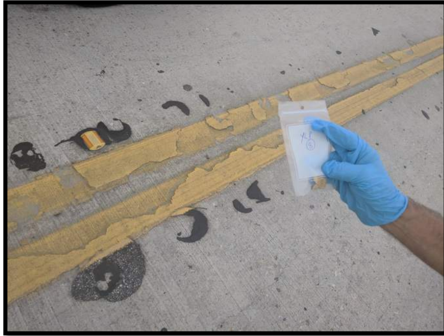
Photograph 9 View of Asbestos Homogeneous Area 3 – Yellow Lane Paint – Roadway Deck (Sample Location 8).
