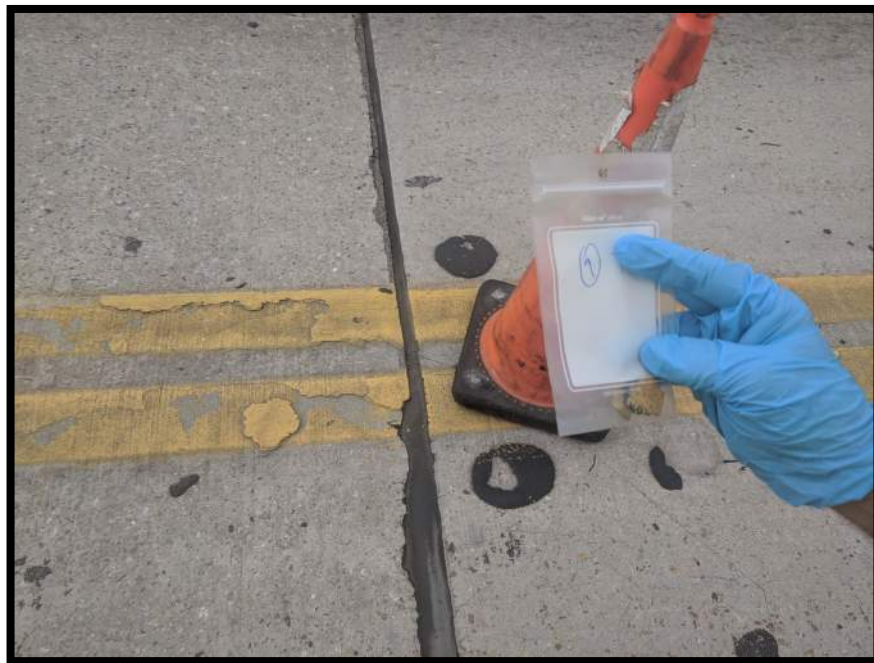
Photograph 10 View of Asbestos Homogeneous Area 3 – Yellow Lane Paint – Roadway Deck (Sample Location 9).
