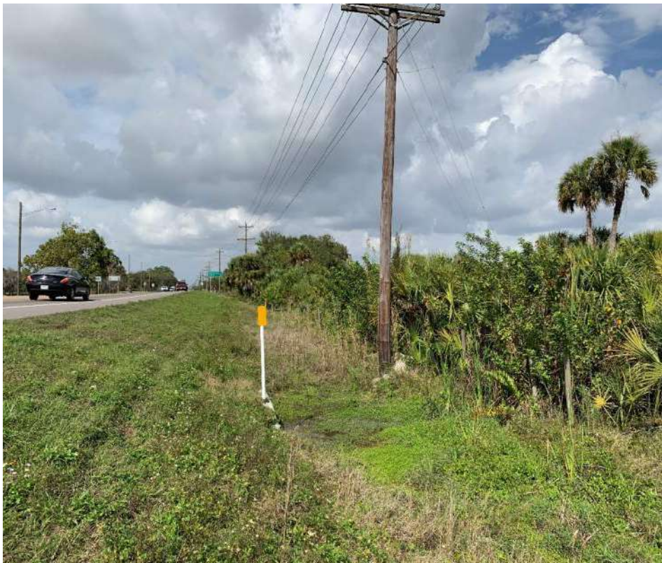
Existing Cross Drain CD-03 – east side of SR 31, Looking North, Downstream Side
