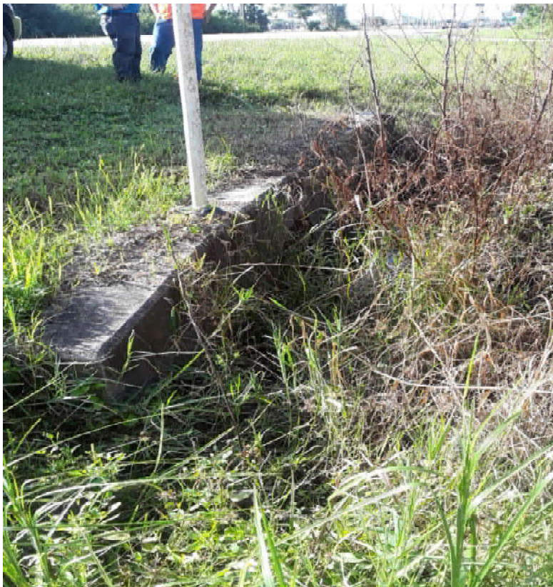
Existing Endwall, Existing Cross Drain CD-01 - West Side of SR 31, Looking South, Downstream Side
