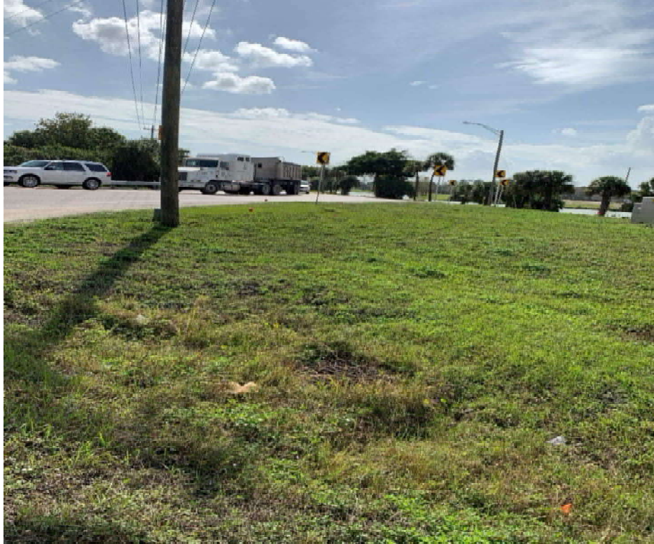
Existing DBI on Cross Drain CD-03 – West side of SR 31, Looking South, Upstream Side
