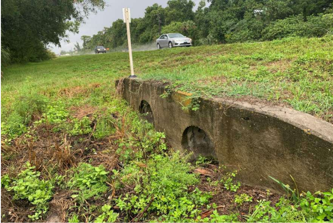
Existing Endwall, Existing Cross Drain CD-01 – West Side of SR 31, Looking North, Downstream Side
