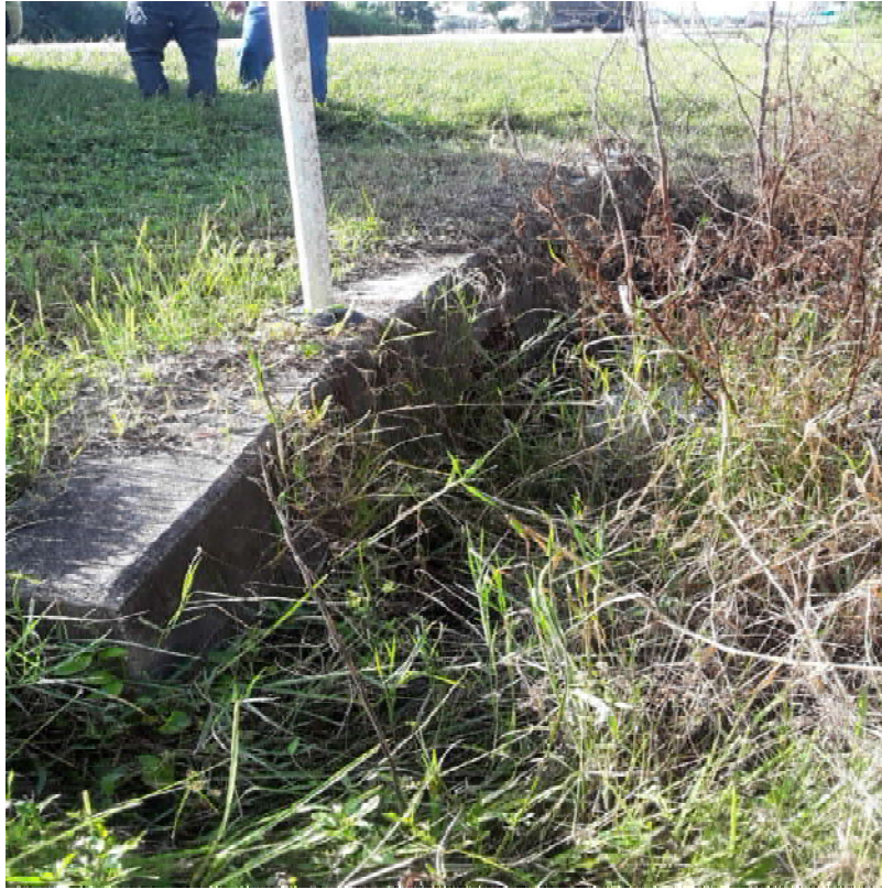
Existing Cross Drain CD-02 – East side of SR 31, looking North, Upstream Side
