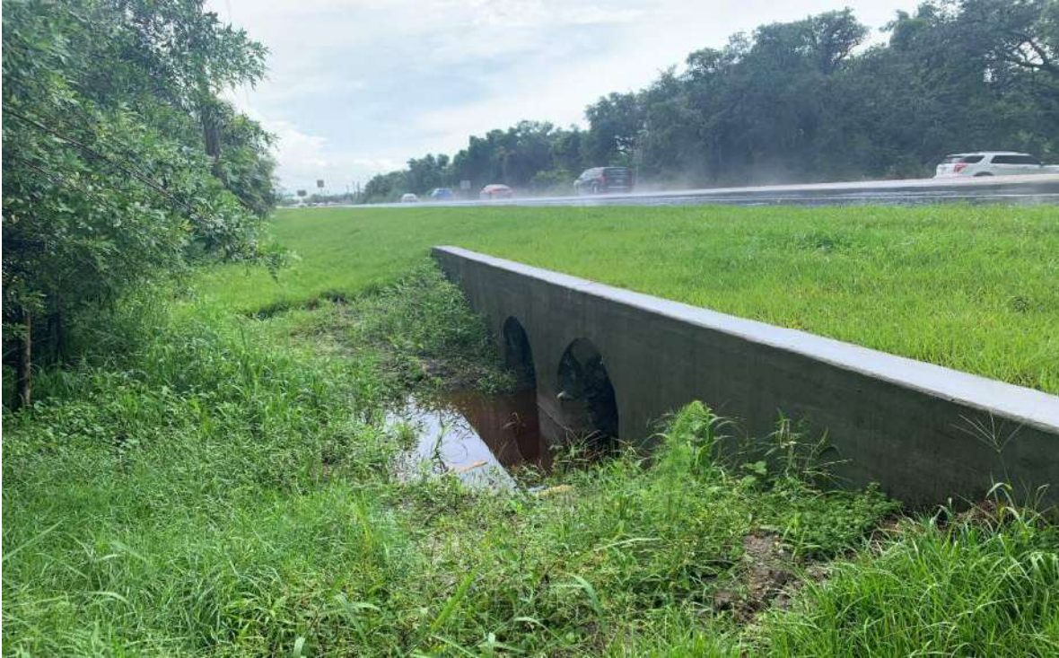
Recently Extended Cross Drain CD-01 – East Side of SR 31, Looking South, Upstream Side
