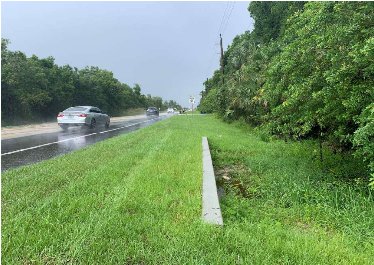
Recently Extended Cross Drain CD-01 - East Side of SR 31, Looking North, Upstream Side
