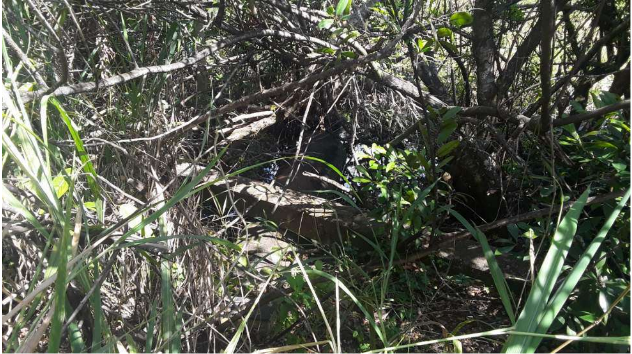
Looking East at Concrete cased Gas Line at location of gas Line crossing Creek
