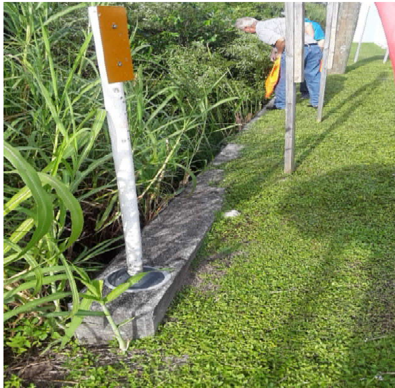
Existing Cross Drain CD-02 – West side of SR 31, Looking West, Downstream Side
