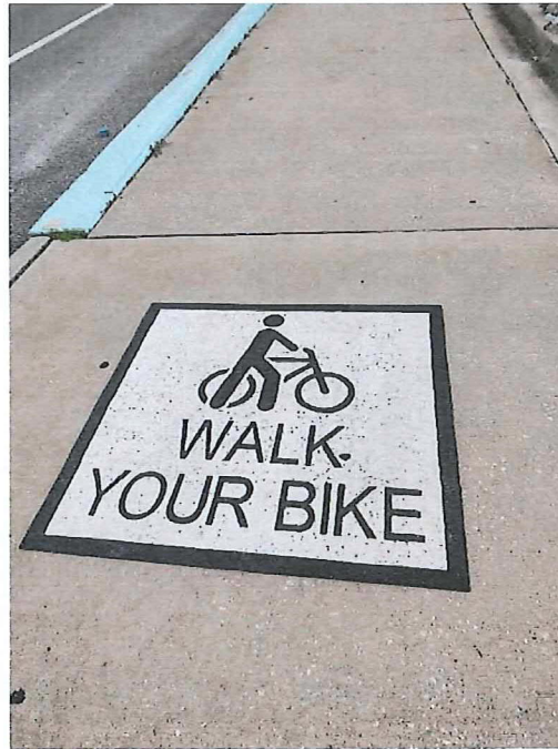
Photo 3. Pavement marking on sidewalk (Estero-Bonita “trail”) at the south end of the Matanzas Pass Bridge
