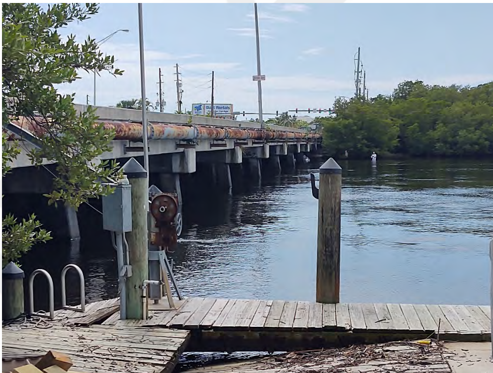
Photo 2. Looking south along the west side of the Hurricane Bay Bridge at Great Calusa Blueway Paddling Trail crossing location under bridge.
