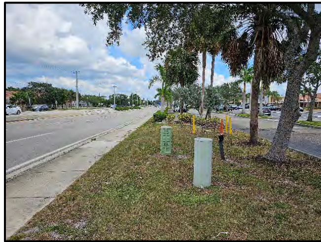
Photo 2.3. Utilities on eastbound ROW of Bonita Beach Road on southeast corner of intersection facing east.
