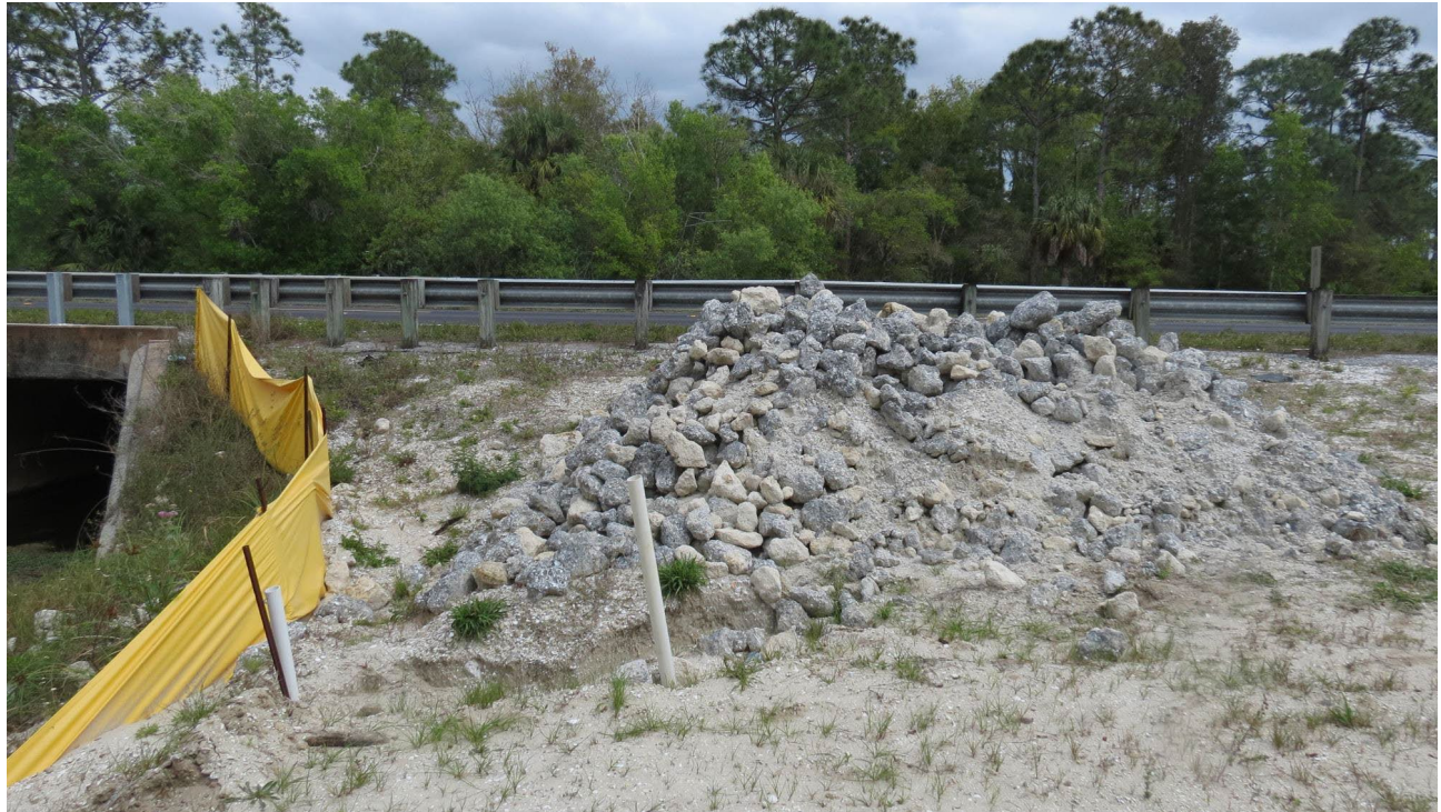
Photo 26. Facing east from ROW at culvert south of Charlee Road. Rubble pile – possible rip rap for culvert work.
