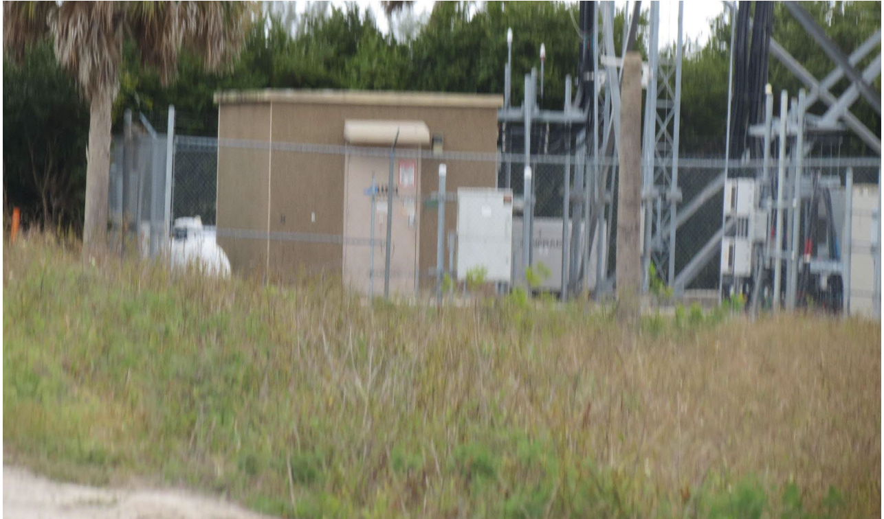
Photo 11. Contamination Site #2: Cell tower area on north side of Burnt Store Road Recycling property. Small propane tank appears to be the fuel for emergency backup generator (not visible).
