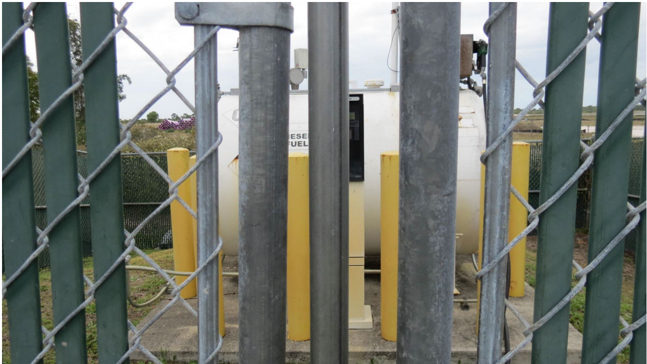
Photo 22. Contamination Site #4: 500-gallon diesel tank for refueling vehicles. Tank is double walled with no visible staining.
