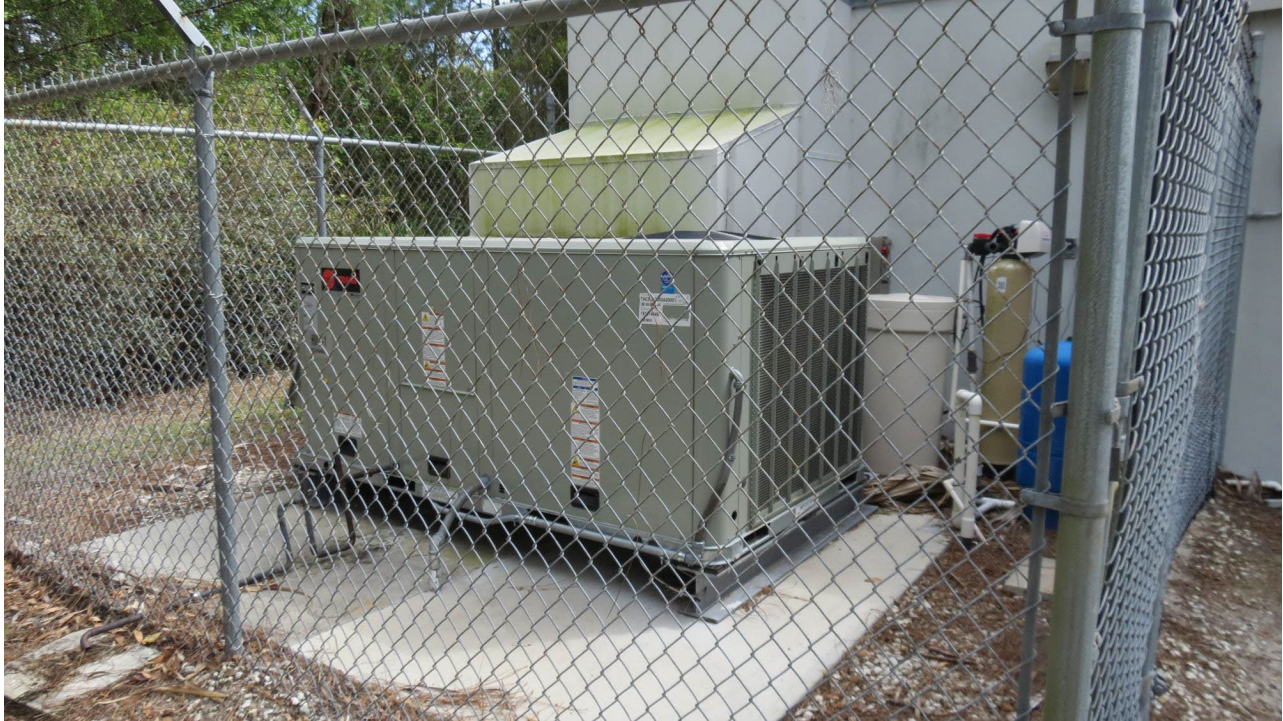
Photo 29. A/C unit for Lumen building. No apparent emergency generator visible on site.
