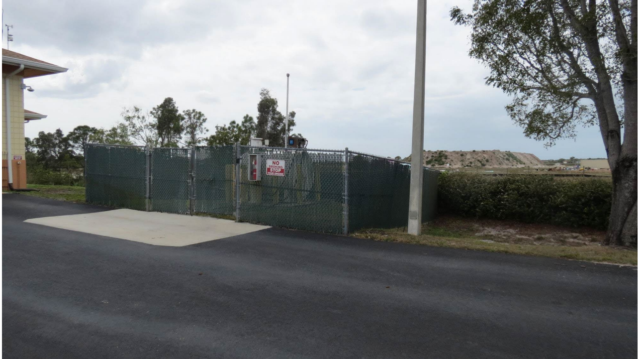
Photo 23. Contamination Site #4: Locked enclosure for diesel AST.
