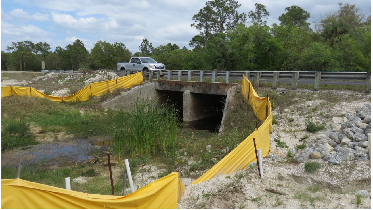
Photo 27. Facing northeast toward Burnt Store Road at box culvert south of Charlee Road.
