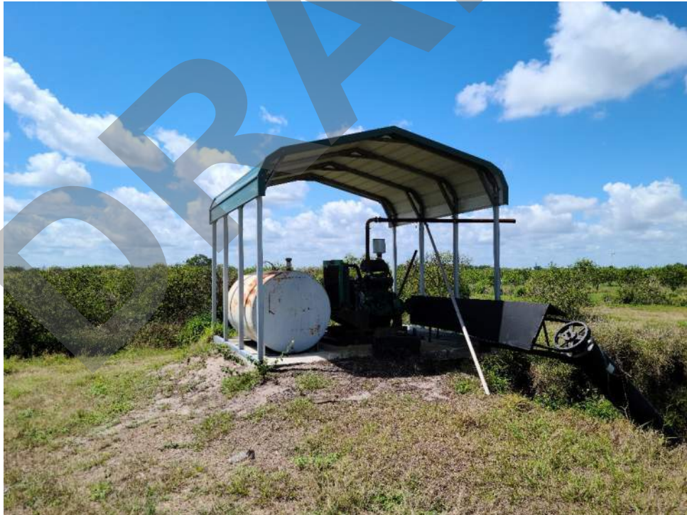
Irrigation pump with diesel AST South of FPC 2A looking south
