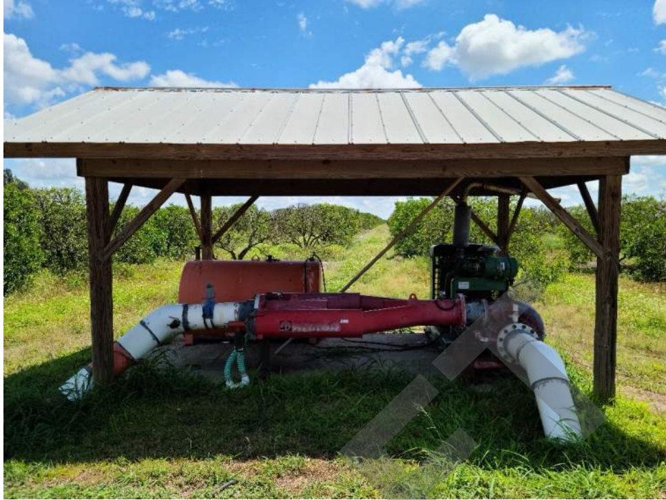
Irrigation pump with diesel AST East of FPC 2A looking east
