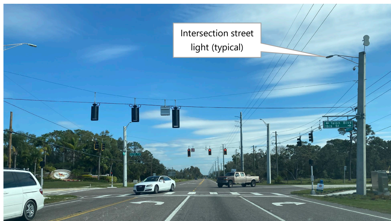
Figure 18: Photo of Lighting on SR 72 at Ibis Street/Talon Boulevard (looking east)
