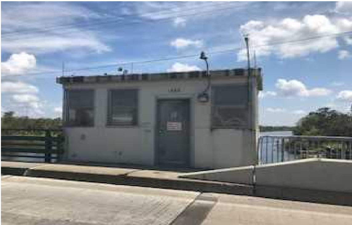
Photo No. 6: View of Bridge Tender House with Non Asbestos-Containing Exterior Stucco
