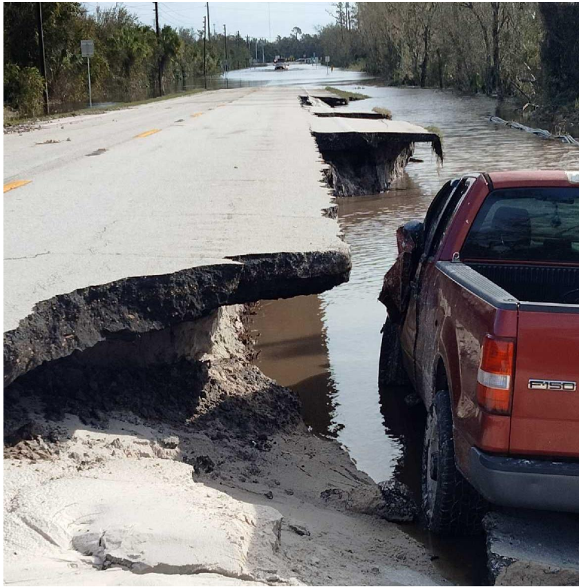
Figure 8–Damage to SR 72 due to Hurricane Ian
