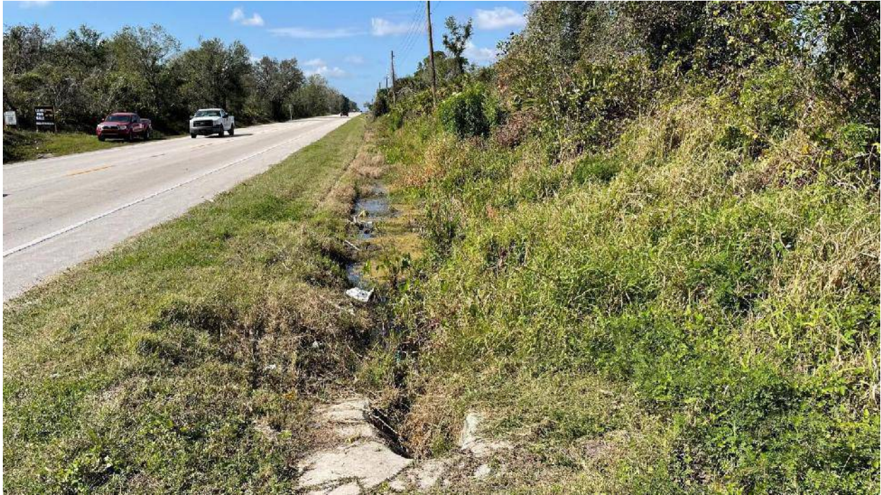
Photo 17 – view southwest toward OSW 2 (FLUCCS 5100), an upland cut roadside ditch in the SR 72 ROW. The ditch contained standing water and litter at the time of review.
