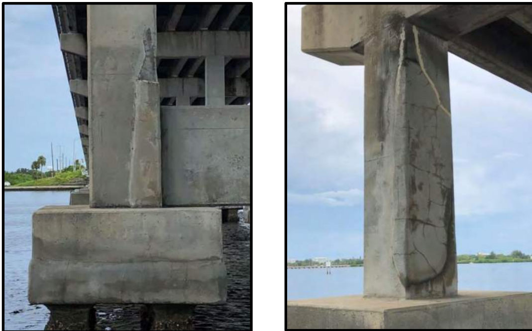
Figure 6. Examples of column repairs that were assigned a condition rating of 2.
