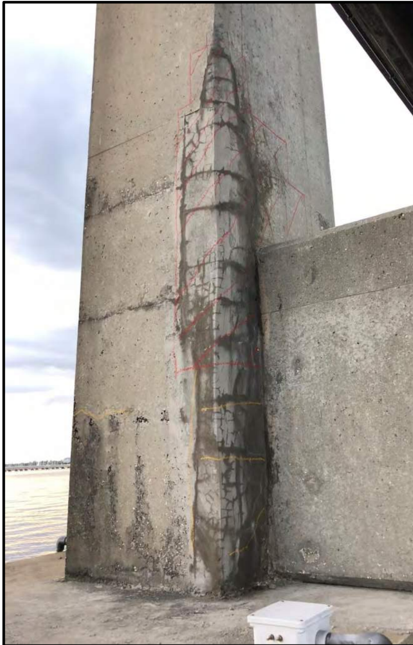
Figure 10. Patched area at the southeast corner of Column 15-1 (delaminated areas are crosshatched in red and larger cracks are highlighted in yellow).
