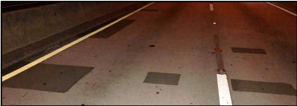
Figure 3. Typical patches on the top surface of the deck.
