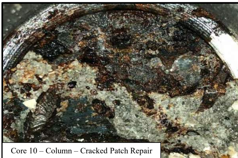
Figure 13. Condition of the reinforcing steel in Column 15-1.
