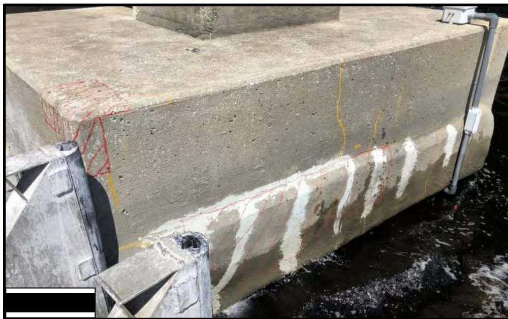
Figure 11. Conditions found on Footing 26-3 (delaminated areas are crosshatched in red and unsealed cracks are highlighted in yellow).
