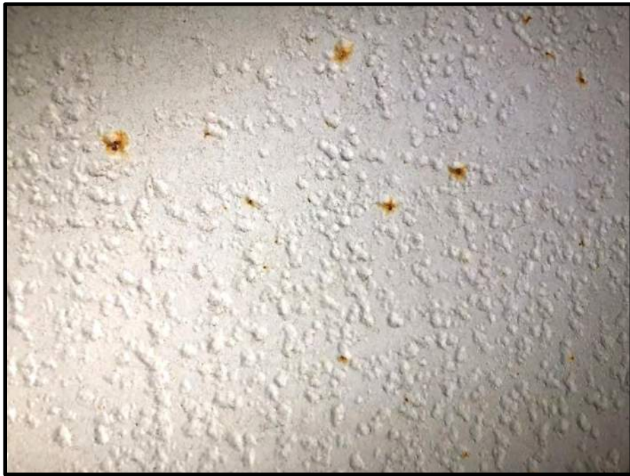
Figure 5. Apparent corrosion products under the coating on a steel beam in Span 18.
