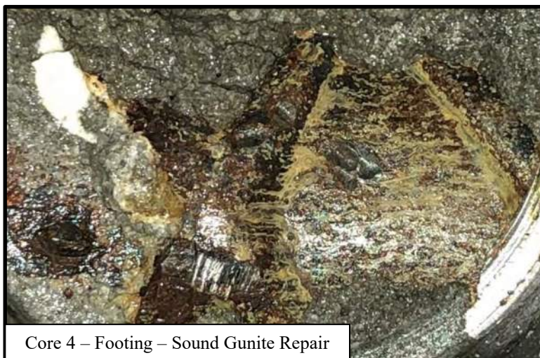
Figure 14. Condition of the reinforcing steel in Footing 26-3.
