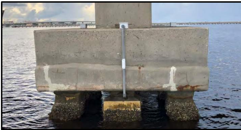
Figure 7. Examples of footing repairs that were assigned a condition rating of 2.
