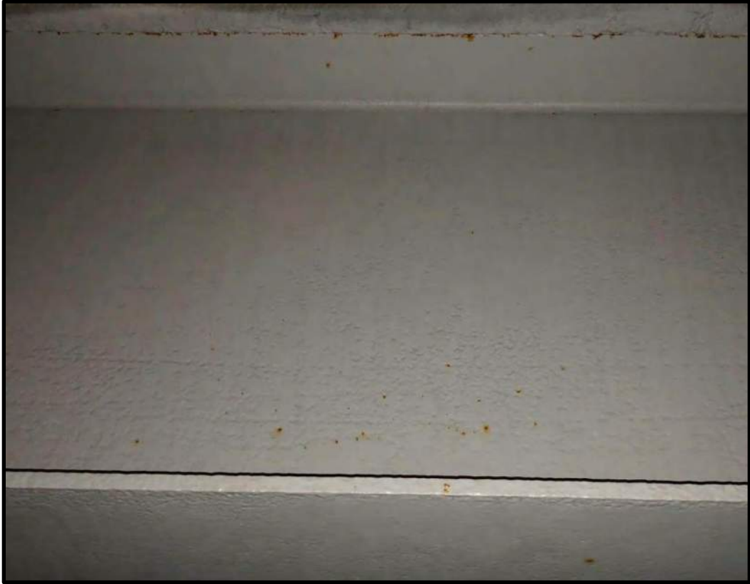
Figure 4. Typical pitting and corrosion staining on a steel beam in Span 18.
