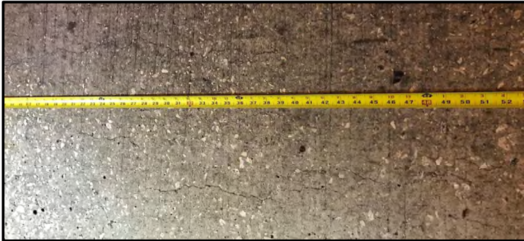
Figure 2. Typical cracking on the top surface of the deck.
