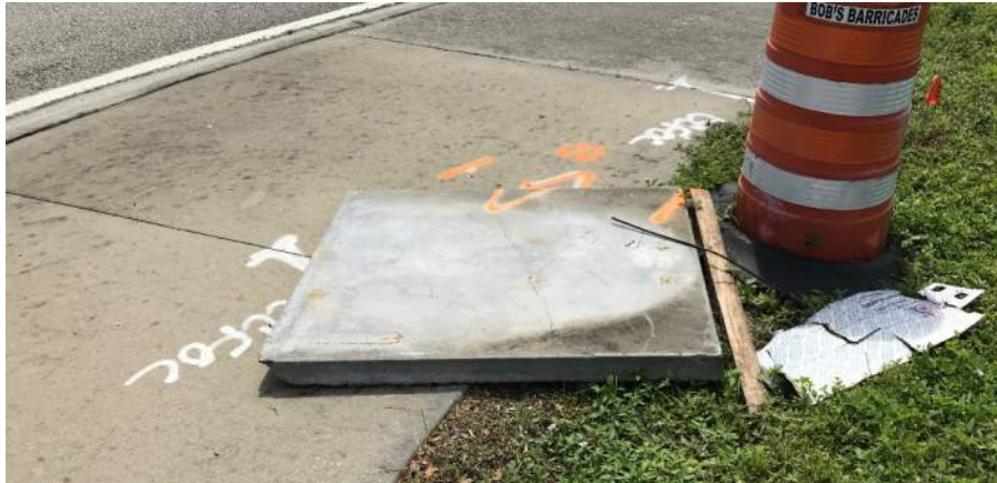
Figure 19: Construction Waste on Sidewalks at SR 78 and Del Prado Blvd
