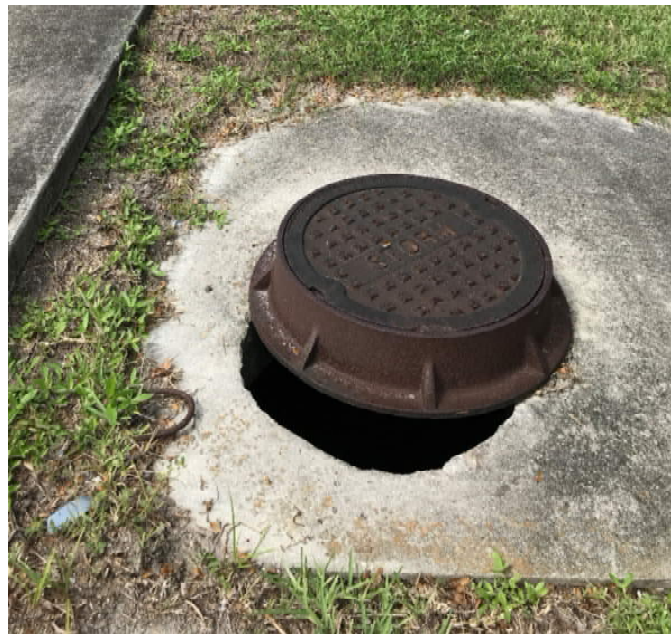
Figure 20: Hole in Slab Around Manhole on Northbound Pondella Road Approximately 280 feet south of SR 78
