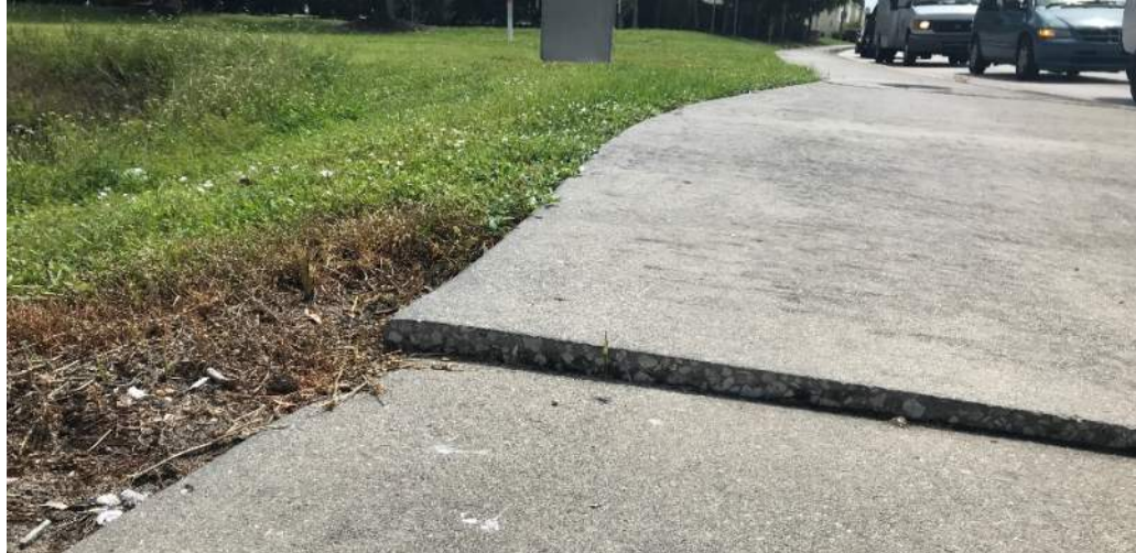
Figure 21: Sidewalk Concrete Slabs Not Flush at the Southeast Corner of SR 78 and Del Prado Boulevard
