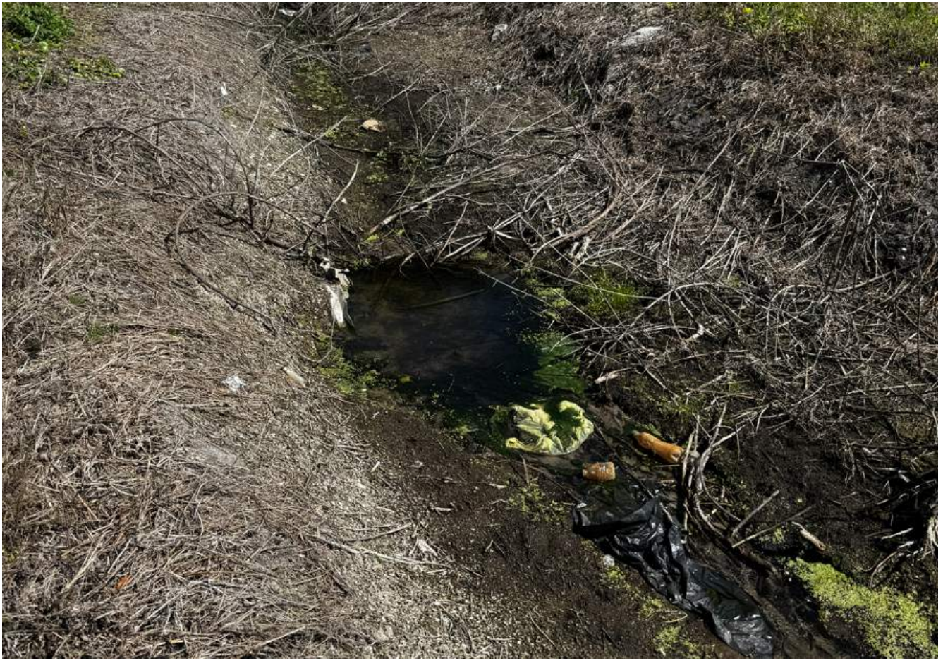
CD-5 30" at US 41 station 258+21 facing north Submerged pipe with no outfall structure
