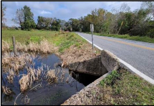
Photo 11 - Looking east at culvert and ROW in APE boundaries on Lake Alfred Road.
