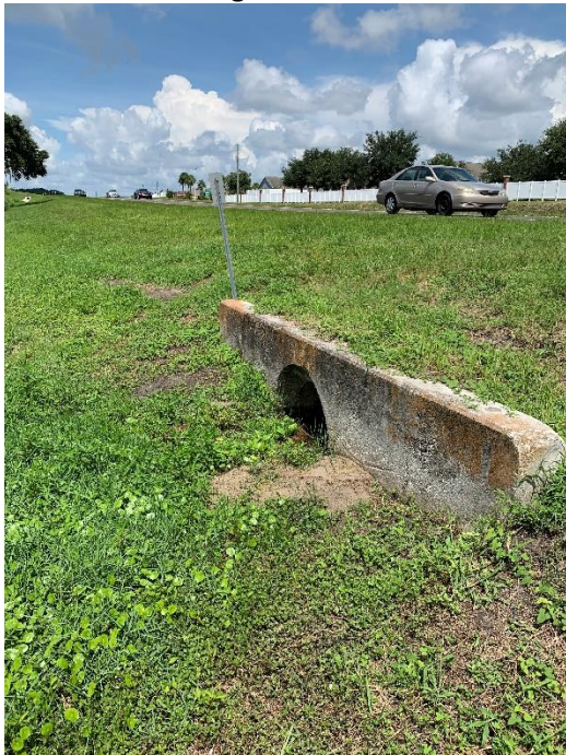
CD 12-17 US 17-92 approx. 200-ft west of Watts Dairy Road Single 18" RCP
