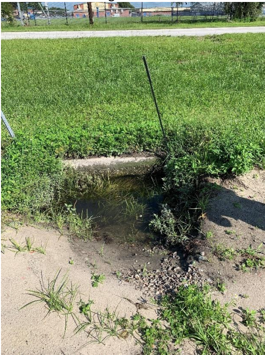
CD 01-03 Along Stadium Road adjacent to Lake Auburndale Senior High School track and field. Single 18" RCP
