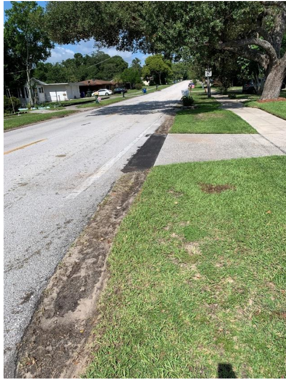
Potential recent underdrain installation on the north side of W Pierce Street west of N Nekoma Ave.
