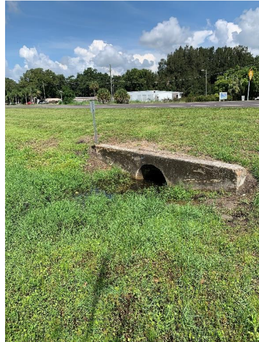
CD 12-12 US 17-92 approx. 1800-ft west of Woodland Drive Single 24" RCP
