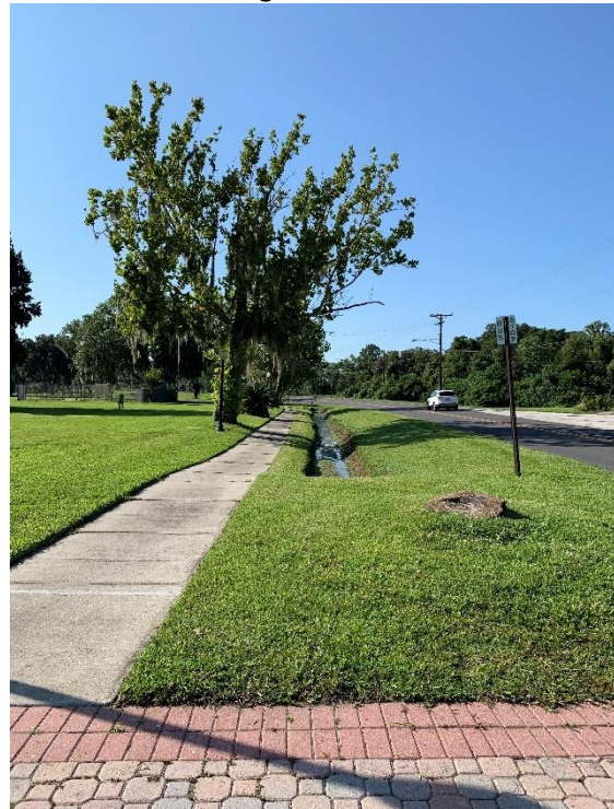
Linear ditch system adjacent to Ramsgate Rd. north of the Lake Ariana Blvd intersection.
