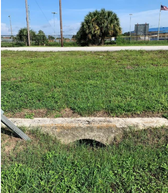
CD 01-01 Crossing Stadium Road approx. 235-ft west of Bennett Street. Single 15" RCP
