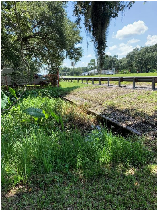
CD 12-13 US 17-92 approx. 300-ft west of Century Drive Single Box Culvert 7' x 6' Concrete
