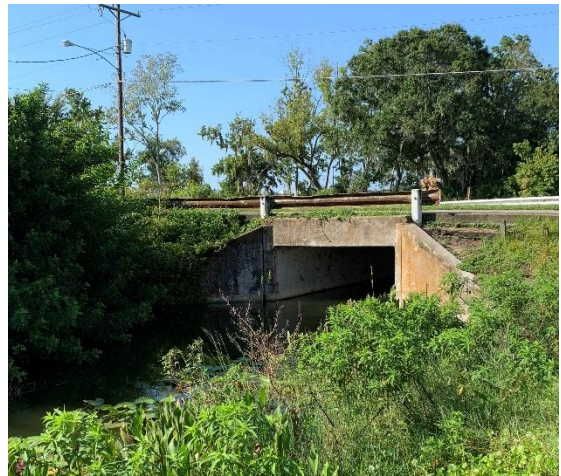
CD 12-08 Ramsgate Road approx. 350-ft northwest of Rafford Road Box Culvert 10.2' x 8.5'
