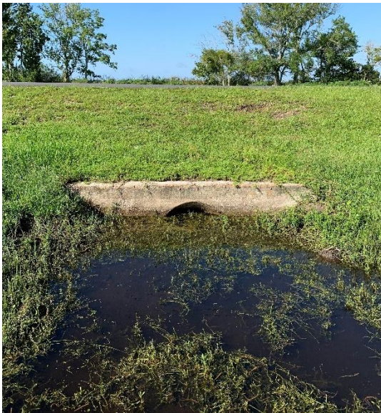
CD 12-07 Ramsgate Road approx. 600-ft south of Lake Ariana Blvd Single 18" RCP
