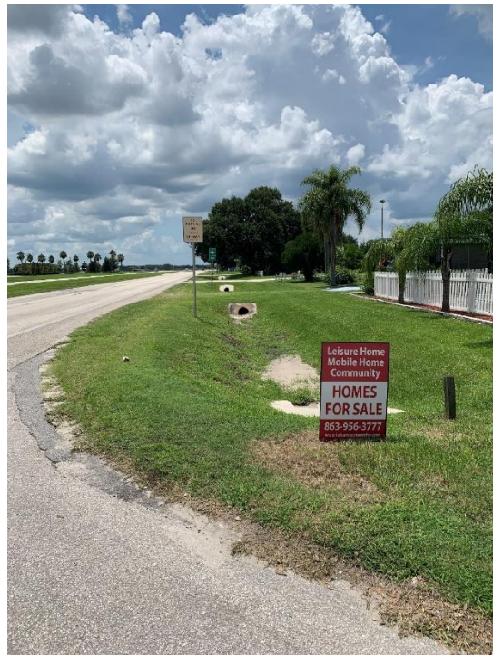
Side drain collection on north side of SR 600 at Idle Lane.
