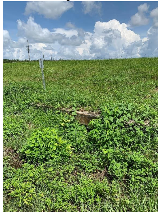
CD 12-14 US 17-92 approx. 1900-ft west of Sweetwater Club Blvd. Single 18" RCP
