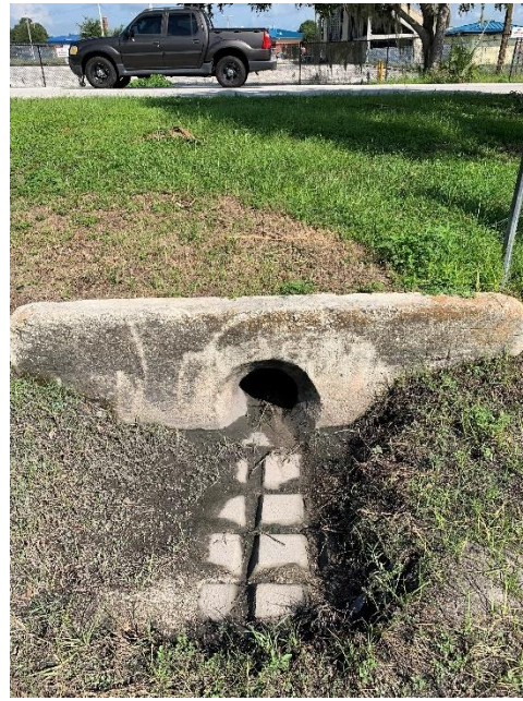
CD 01-02 Along Stadium Road southwest of Lake Auburndale Senior High School track and field. Single 15" RCP
