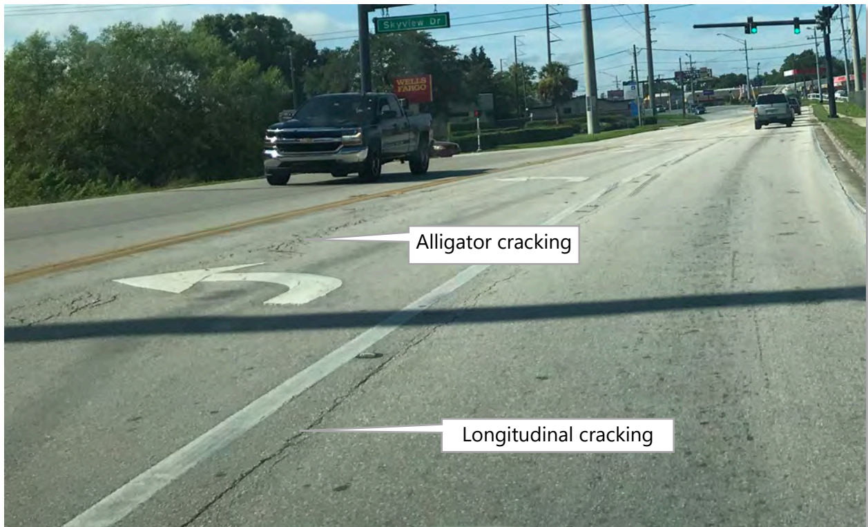
Figure 14: Photo of pavement distress on Combee Road (looking south)
