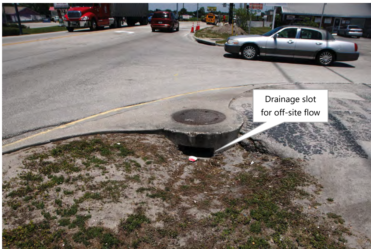
Figure 20: Photo of Combee Road curb inlet at Industrial Park Road (looking north)
