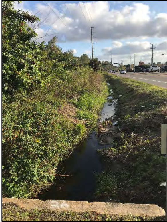
Drainage ditch – located on the east side of Combee Road north of North Crystal Lake Drive.
