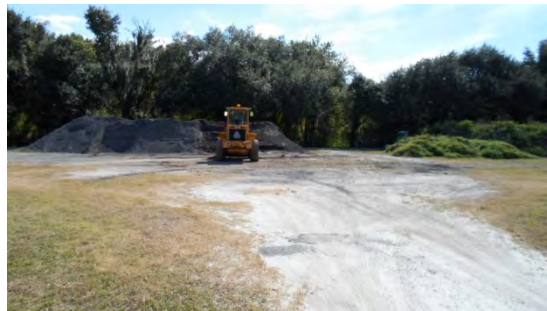
SMF-1: North boundary near entry gate looking south at crushed asphalt and soil stockpiles
