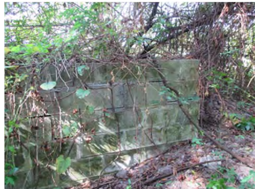
SMF-5: Overgrown concrete block structure approximately 10'x10'x4' near NE corner
