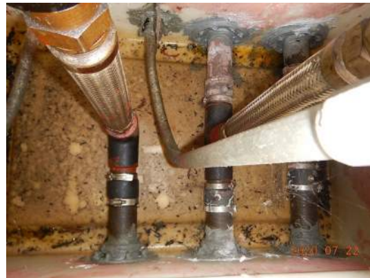
2020-07-22 Typical dispenser sump
