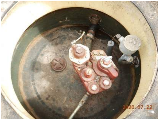
2020-07-22 Typical STP sump & components
